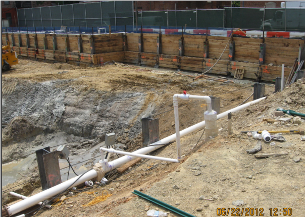
^ Pictured above is the actual excavation of the southern building foundation, compliments of Balfour Beatty Construction.
